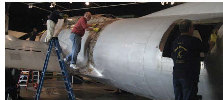
Volunteers removing the "protective" plastic covering that had adhered to the fuselage over 25 years.
